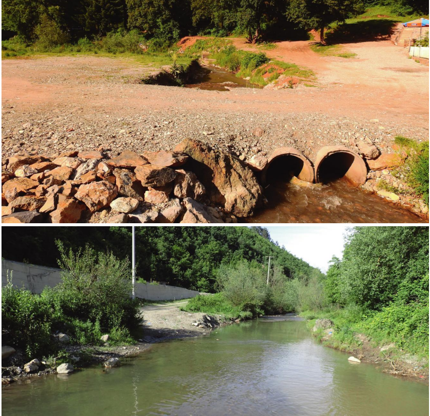
Figure 50: confluence of Reka e vogel (above) and Reka e madhe (below) rivers upstream of Nerodime Village (Loc. 55).
